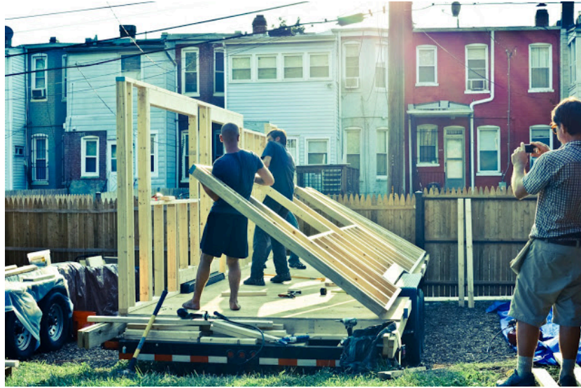
Image: Raising the interior wall of the “Matchbox” tiny home, built on a trailer bed
